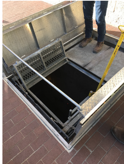
Fig. 4. Entrance to a network vault.
