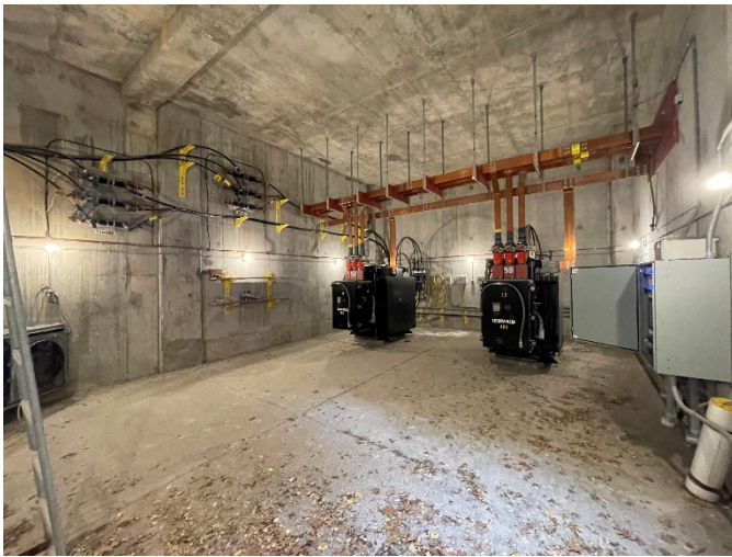
Fig. 7. Inside a large 480 V network vault.
