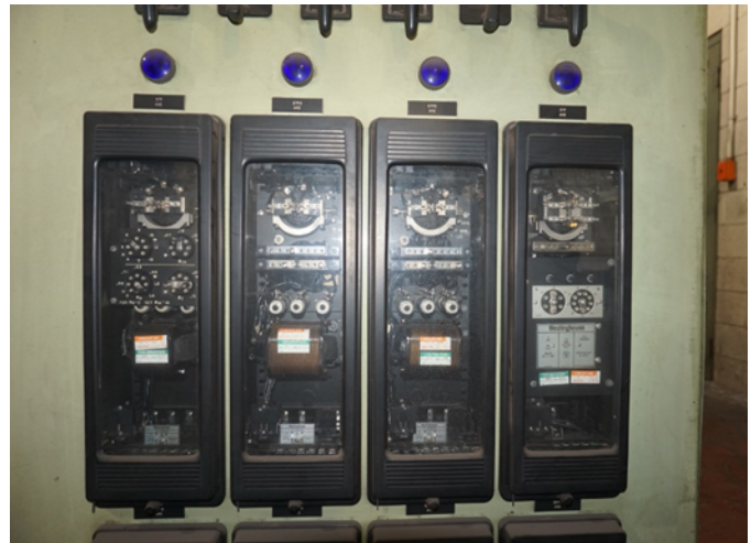
Fig. 3. Previous panel-mounted 138 kV line relays.
