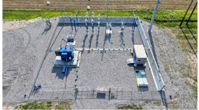
Fig. 1. The 138 kV/34.5 kV DSS substation.
