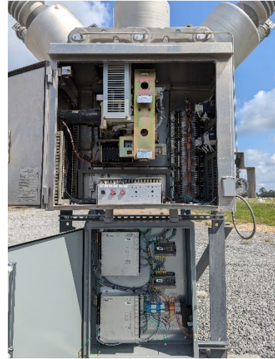
Fig. 3. Rental breaker MU retrofit.
