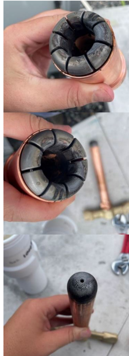
Fig. 15. Bkr 2 damage caused by lightning.
