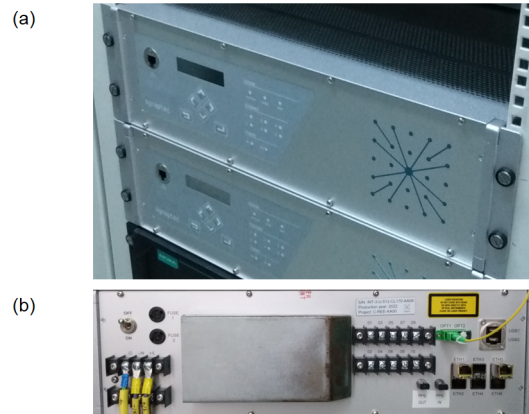
Fig. 4. Interrogator installed in a substation: front (a) and back (b) views.
