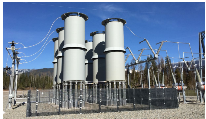
Fig. 2. A three-phase dry-type air-core shunt reactor (238 kV, 50 MVAR).
