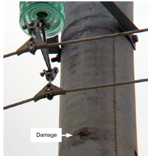
Fig. 23 Flashover damage on concrete pole
