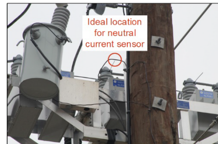
Fig. 1. Typical pole-top capacitor bank installation (a) and close-up of a neutral conductor from the wye point to the ground (b)
