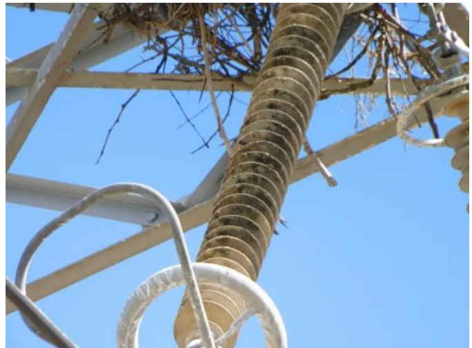
Fig. 11. Evidence found of the December 17, 2019, fault, showing bird contamination and arcing across the insulators.
