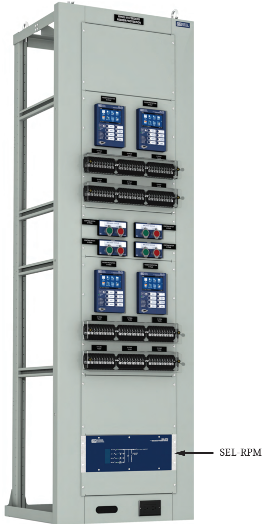
Figure 4 SEL-RPM Installed in a Panel
