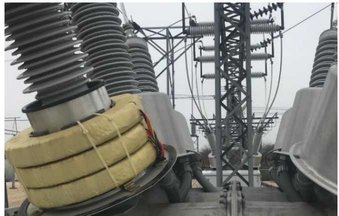
Fig. 11. Cover of Pole 1 removed.
