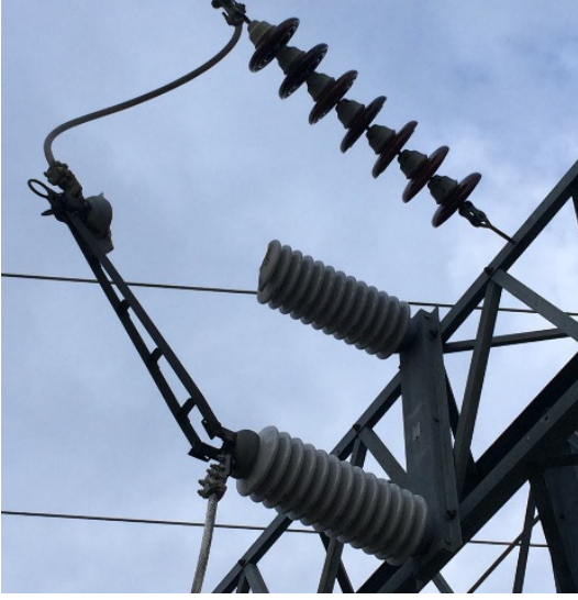
Fig. 5. First fault on A-phase of Switch S11.
