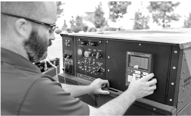
Fig. 3. TQG After a Controls Upgrade
