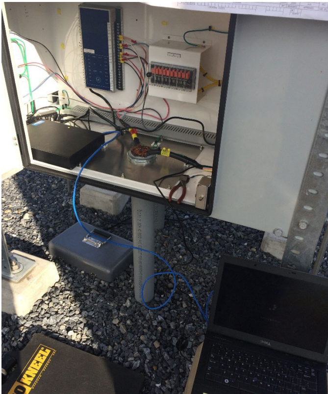
Fig. 8. DAQ device installed in the breaker at the PPL substation.
