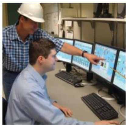
Central control room.
