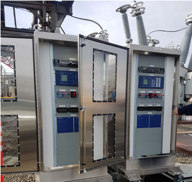
Fig. 38. Mobile Relay Panels
