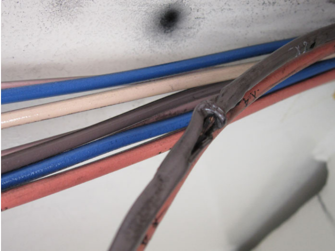
Fig. 14. Arcing to the tank and punctures on CT secondary insulation
