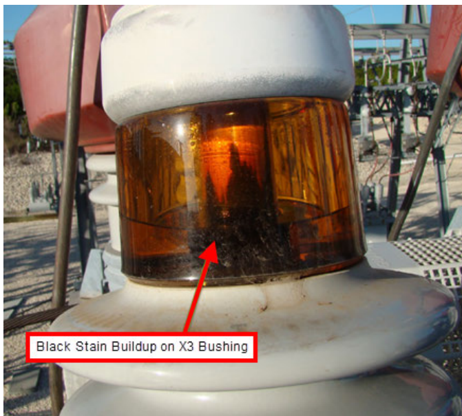
Fig. 9. Black stain buildup observed through the sight glass of the X3 bushing
