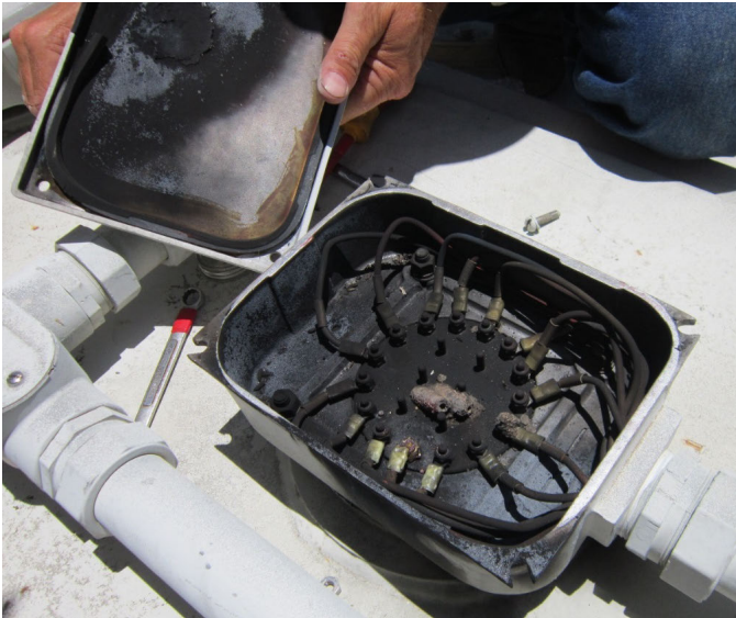
Fig. 15. Damage to high-side Junction Box 1
