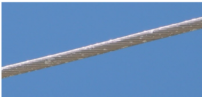
Fig. 14. Pitting and Beading on Conductor Following Phase-to-Phase Contact
