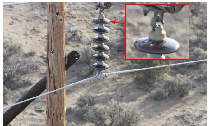
Fig. 12. Flashed-over insulator on the C-phase, tower 8/6 (eighth tower after the sixth mile) of the Brasada-Harney line.
