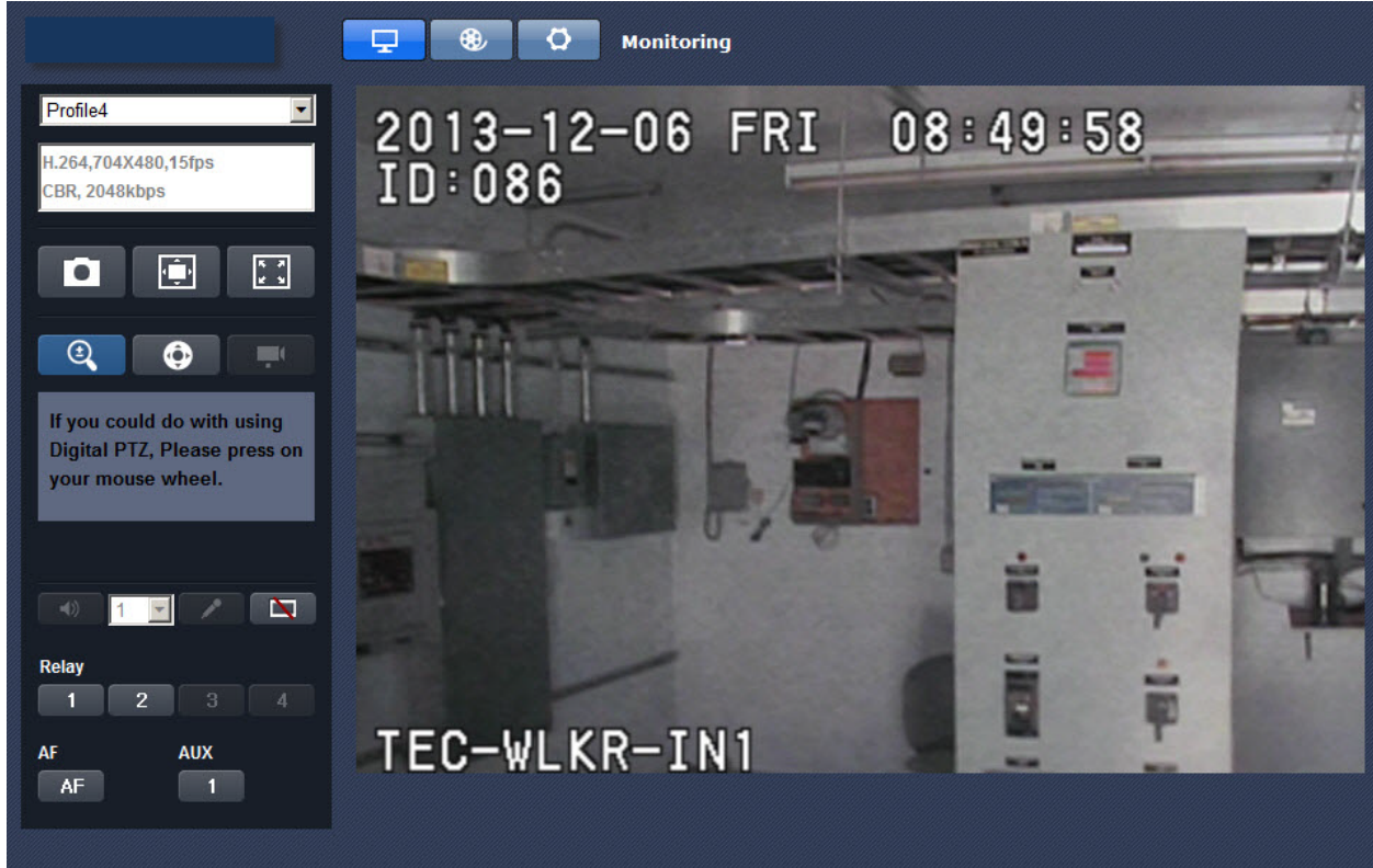
Fig. 13. Substation interior video image.
