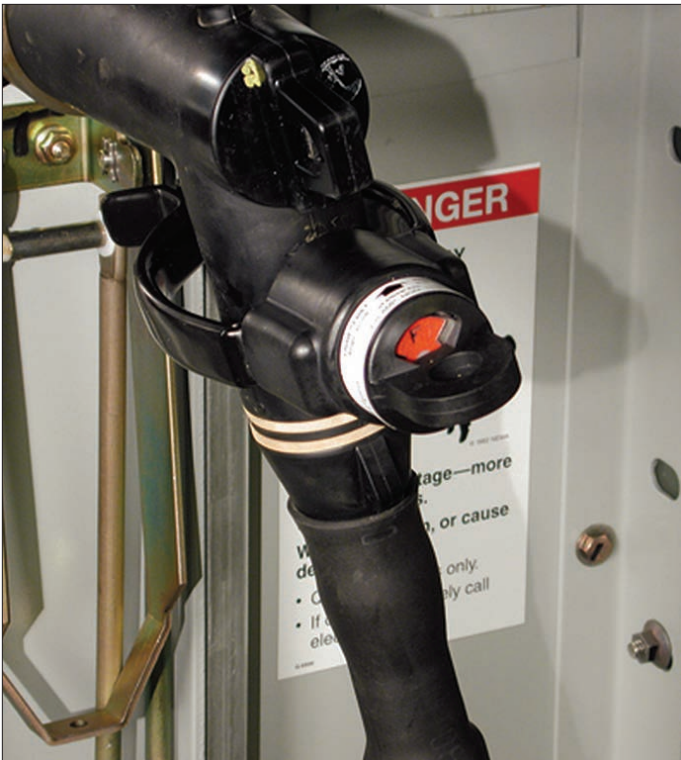
A Test Point Reset Fault Indicator with junction shield provides indication in a switchgear cabinet.
