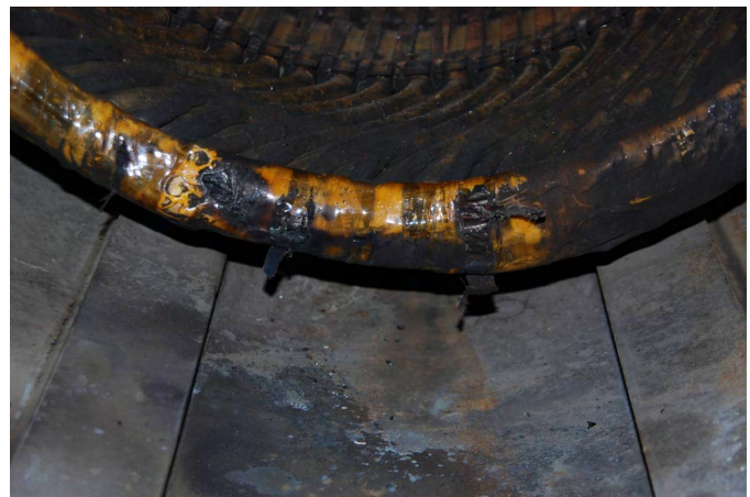
Fig. 43. Generator Fault Damage
