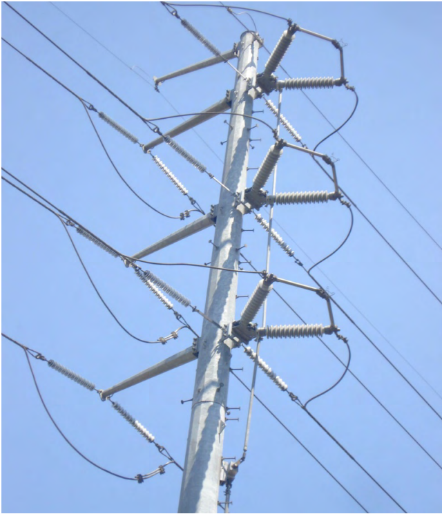
Fig. 2. View of the 115 kV MOD switch on the PEGI I-NYLON line (Switch 89C in Fig. 1).
