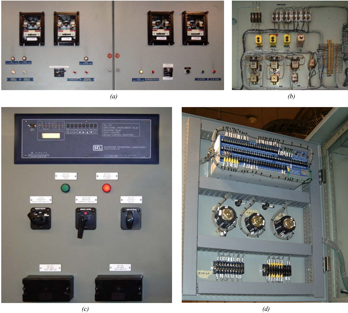
Figure 4—This transfer scheme project replaced electromechanical relays and pneumatic timers, which are known to have a limited life cycle (a and b). The new microprocessor-based protective relays provide more functionality and increased reliability (c and d).
