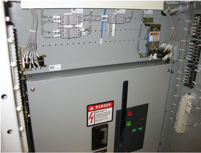
Fig. 8. Lens sensor installed above breaker
