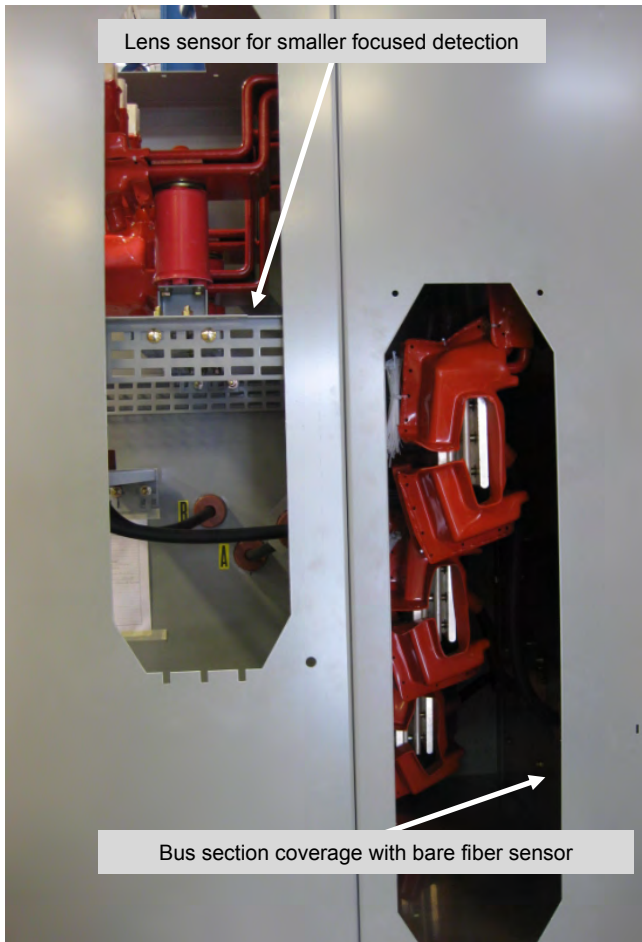
Fig. 9. Typical installation locations for arc sensors
