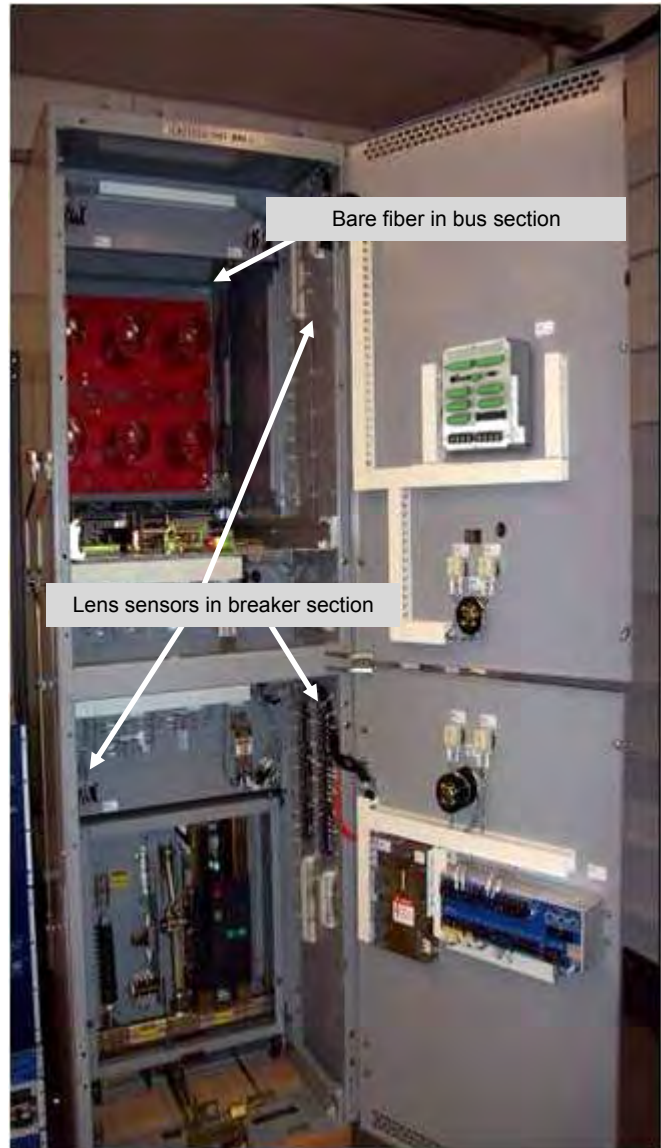
Fig. 7. Install sensors in bus breaker input and output sections
