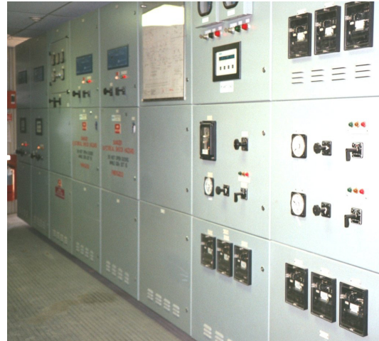
Figure 2—With a history of unreliable power service and paper maintenance records showing 1,000 trips on the utility tie breaker for a total of 24 hours of power outage, the priority was to reduce the trip index and increase power reliability to the plant.
