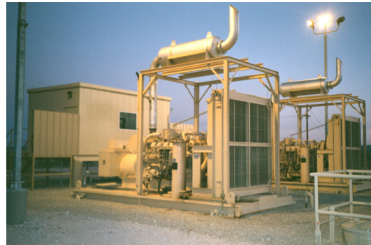
Figure 1—Most large oil and gas facilities maintain on-site power generation, with their connection to the utility grid serving as a backup power source.
